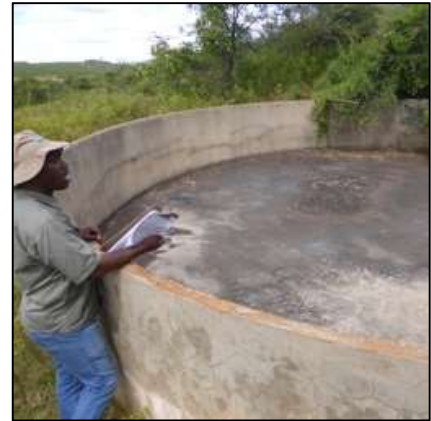
Night storage reservoir
