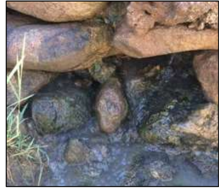
Leak in spillway wall
