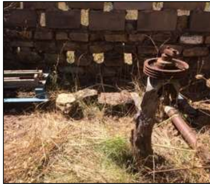
Mono pump – no diesel drive motor
