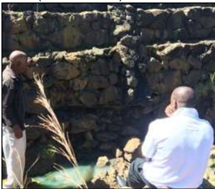
Leak in spillway wall
