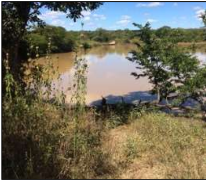
Untapped dam – minor leak
