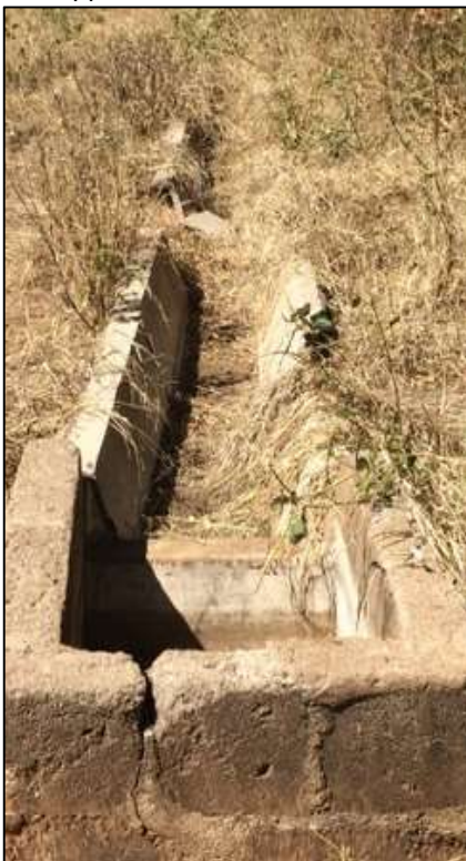
Main canal – needing repairs
